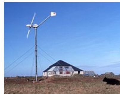
Ground-mounted wind turbine
